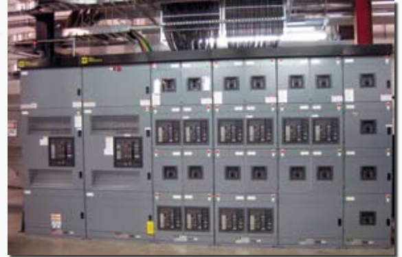
Toshiba UPS Witness Test Facility in Houston, Texas
