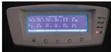
Power consumption trends for up to 23 months can be viewed through a history log - a powerful aid in capacity planning and diagnosis as events are time- and date-stamped as they occur.
