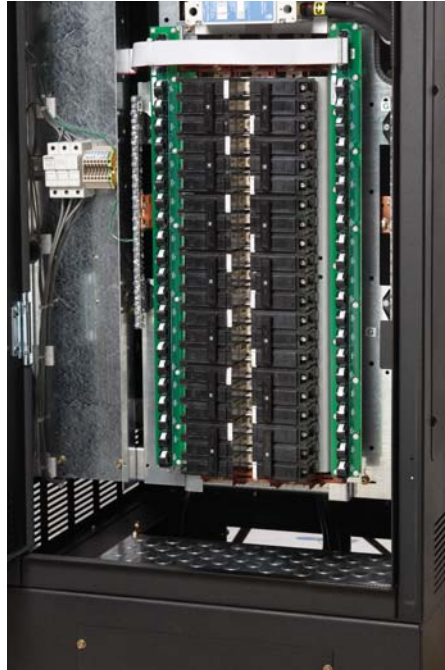
Easily accessible area for bottom cable entry - can be easily rearranged to allow for top entry.
